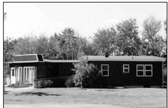
The flat roof on this single-story building is inappropriate, as is the false parapet on the left (front) of the structure.
